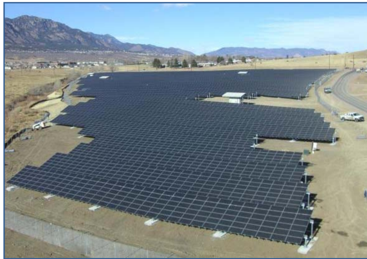
At Fort Carson, Colo., the Army partnered with a local energy provider in an enhanced-use lease. The energy provider built a photovoltaic solar array on top of a closed landfill. That site now provides energy to some 540 homes. U.S. Army photo.
